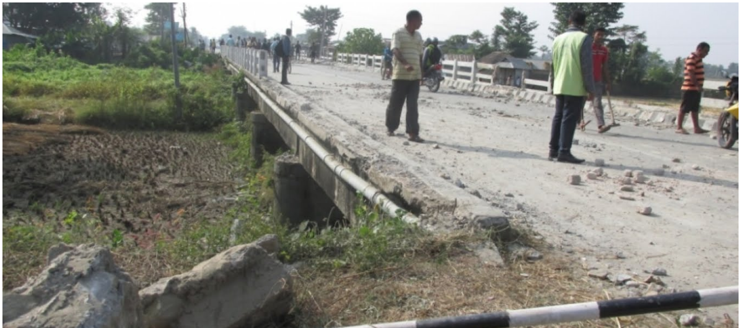
The bridge is damaged but still standing. Image: Bhola Paswan
