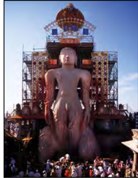
Scaffolding has been constructed around the statue of Bāhubali in preparation of the great ritual.
